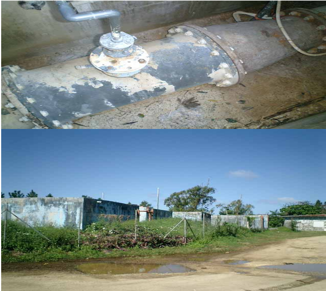
Photo 4 - Chlorine injecting chamber (above), Photo 5 -Concrete reservoirs holding water pumped from the boreholes at Mataki Eua. (Davendra Nath-SOPAC)
