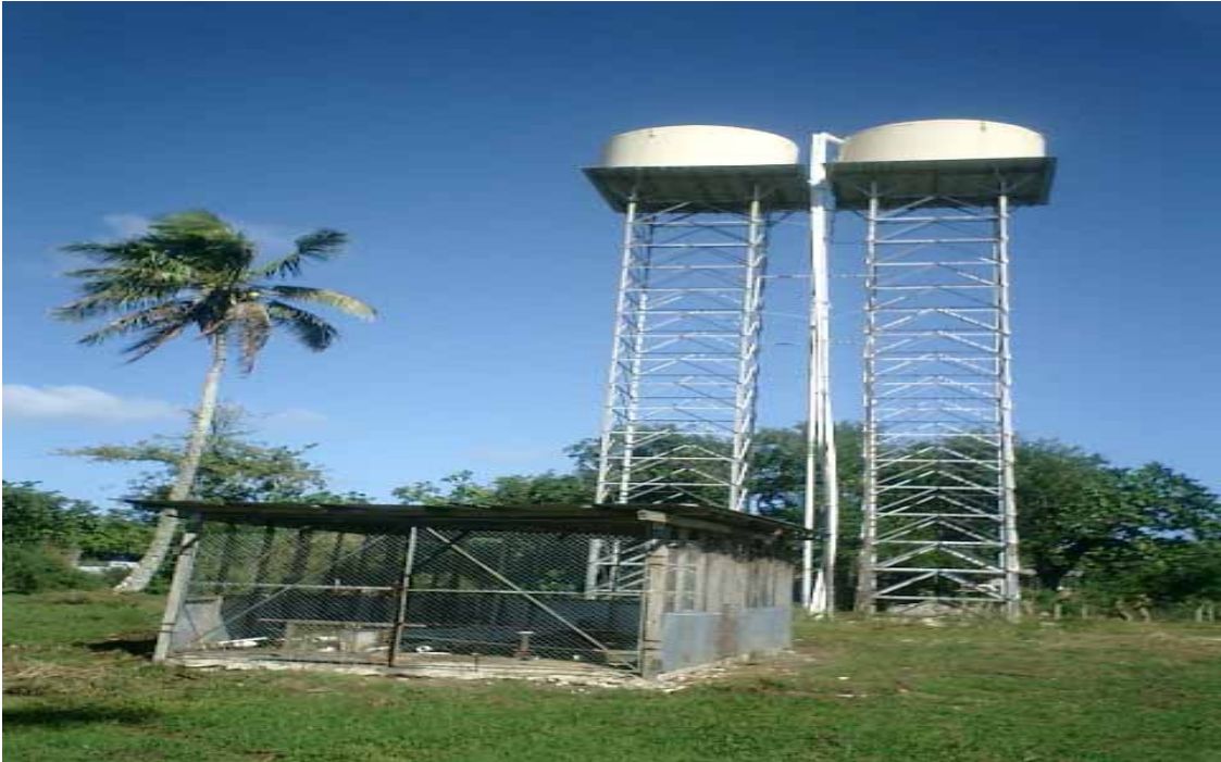
Photo: 6 Elevated header tanks, borehole well shed for Rural Supply system (Davendra Nath-SOPAC)
