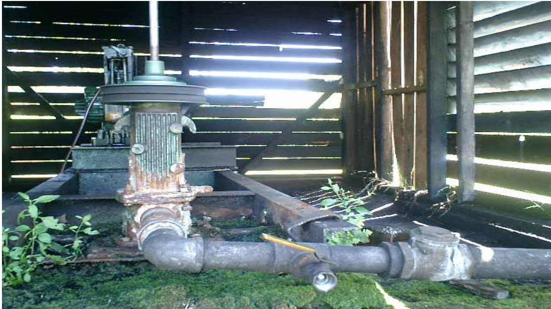
Photo: 2 Borehole overhead mechanical pumps (Davendra Nath-SOPAC)
