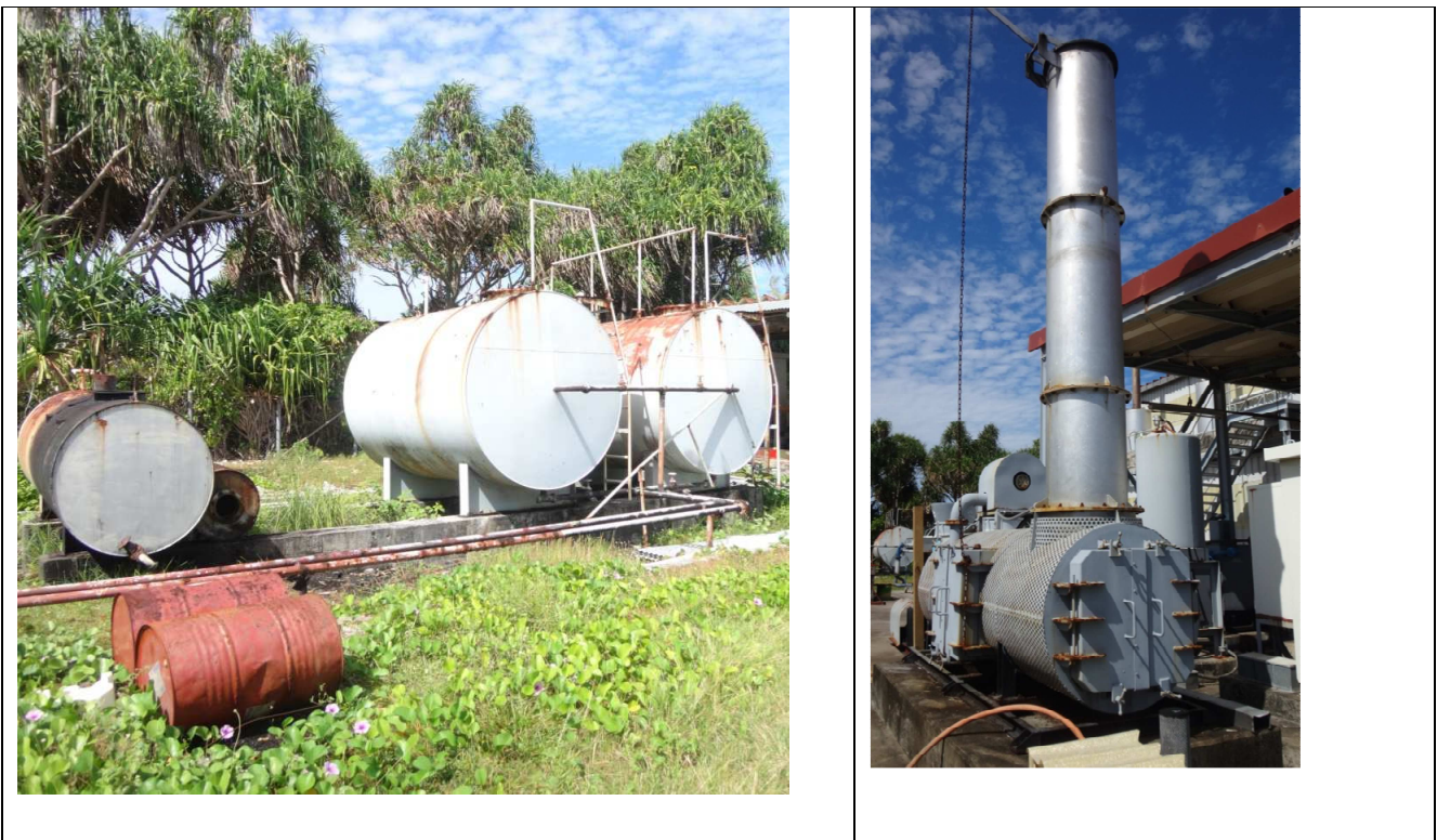
Figure 4: TEC Power Station: Waste Oil Tank –and Incinerator
