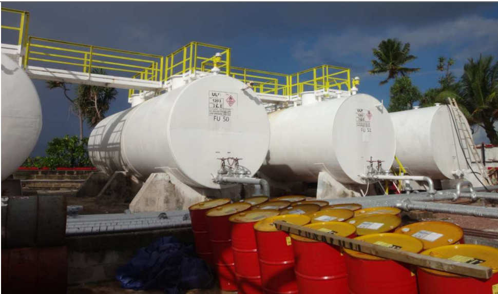
Figure 3: Pacific Energy Storage
