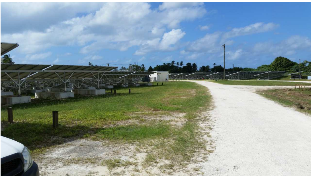
Figure 5: Solar Power at Popua Power Station
