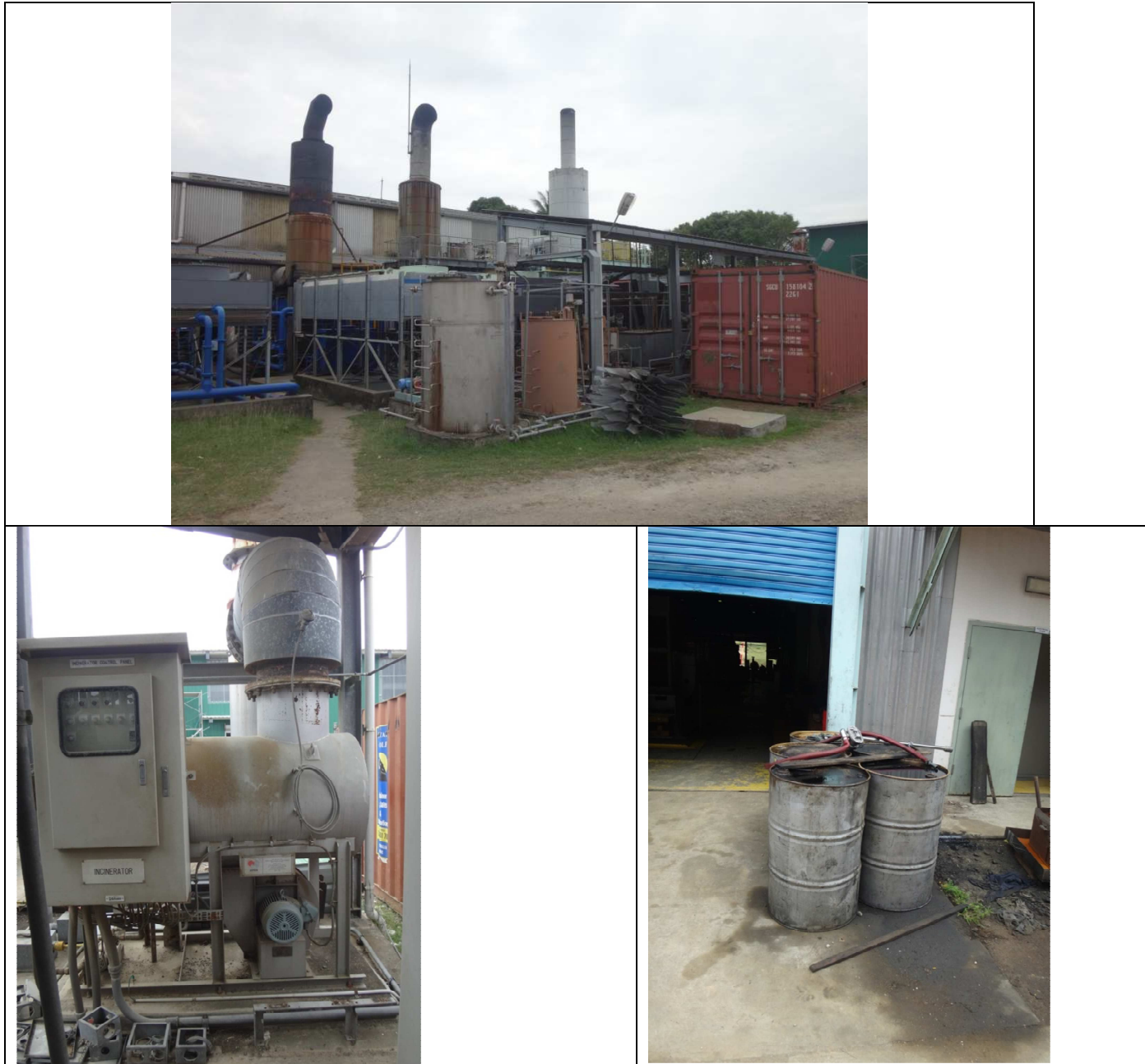
Figure 5: Lungga Power station and Waste oil management
