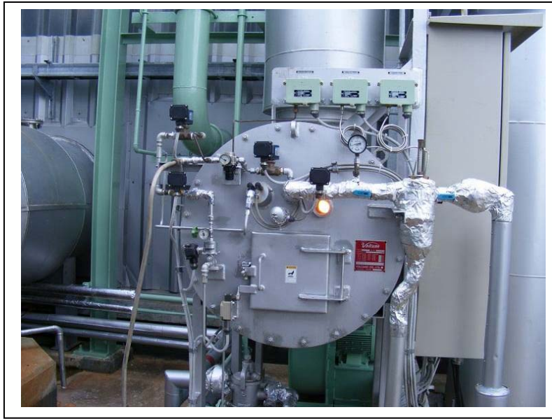
Figure 1 – Aimeliik power plant used oil burner
