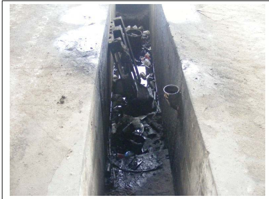
Figure 3 – The inspection pit showing the open pipe connected to an underground storage tank
