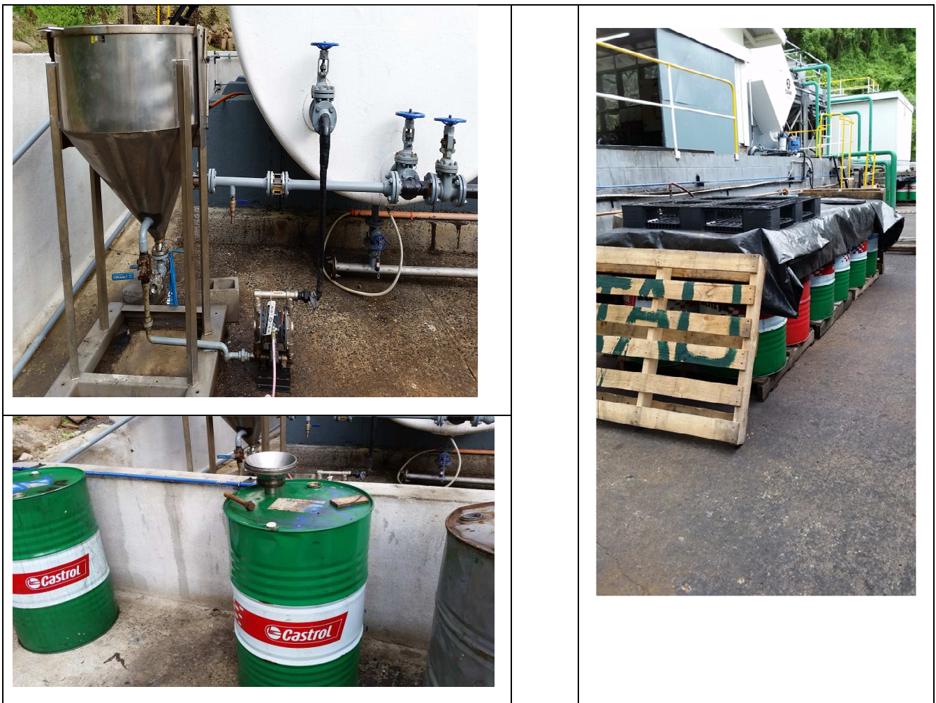
Figure 3: Waste Oil Management at Power Station
