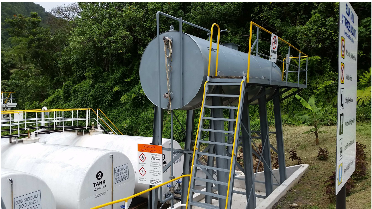
Figure 2: Waste Oil Tank - TAU Power Station
