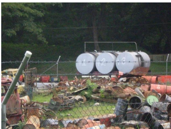
Photo 3 - VGML Waste Oil Storage
