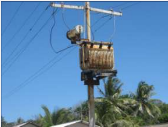
Figure 1. Many of our assets urgently need repair
