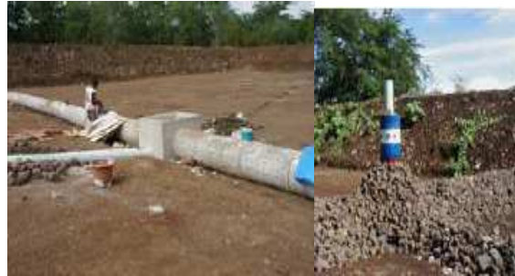
Leachate collection pipe Gas venting pipe
