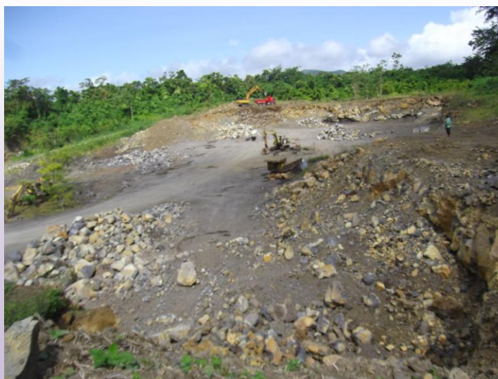
Figure 15: An example of a large scale rock and aggregate mining operation in Samoa - Sale'imoa, Upolu Island. Source: MNRE 2015.
