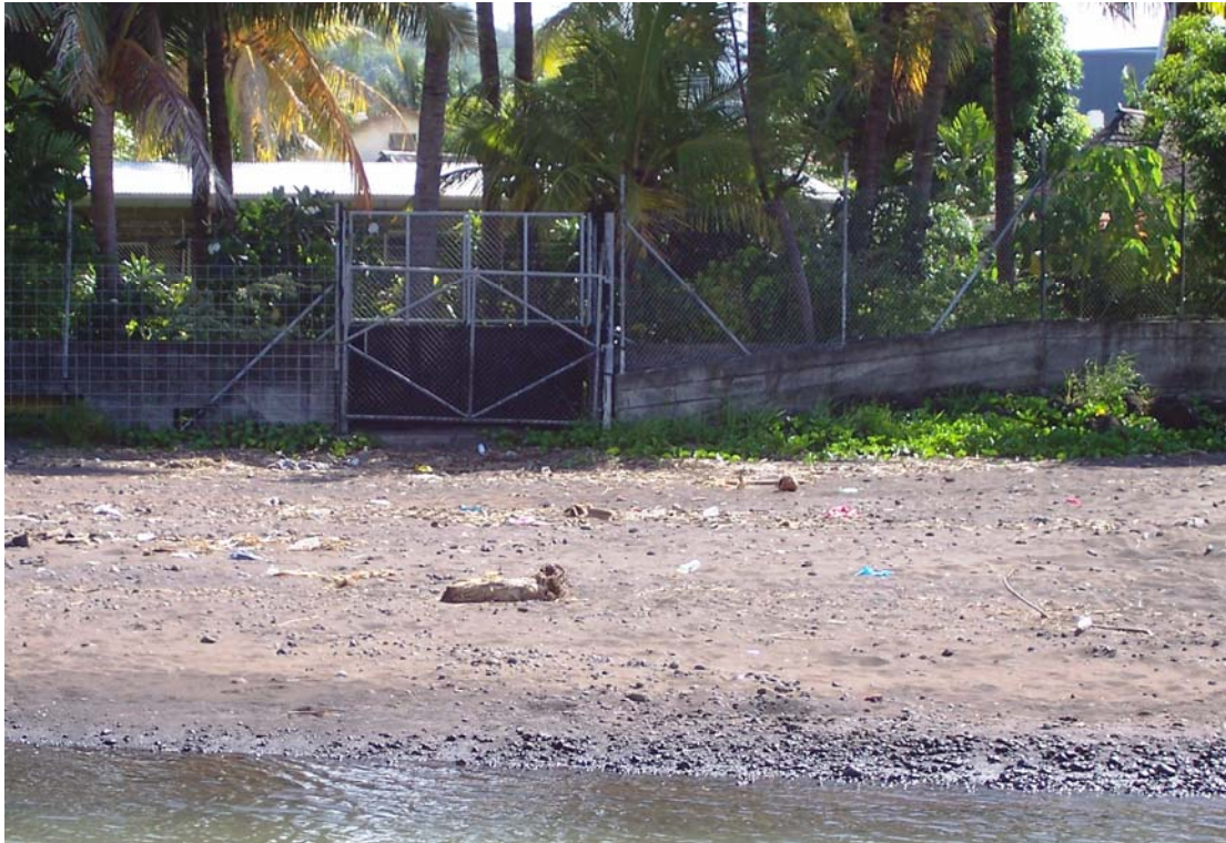
Figure 2-1: Flood wall at Aggie Greys Hotel at the mouth of the Vaisigano
