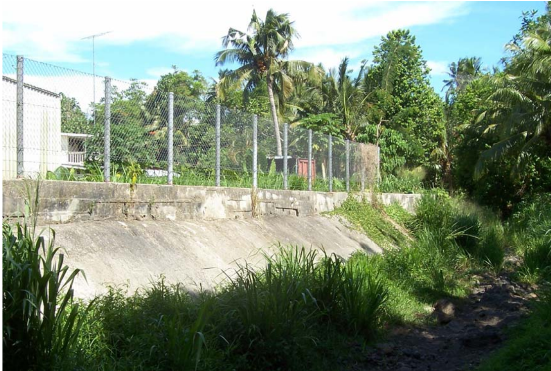
Figure 2-2: Flood wall and bank protection for commercial property on a tributary of the Vaisigano River
