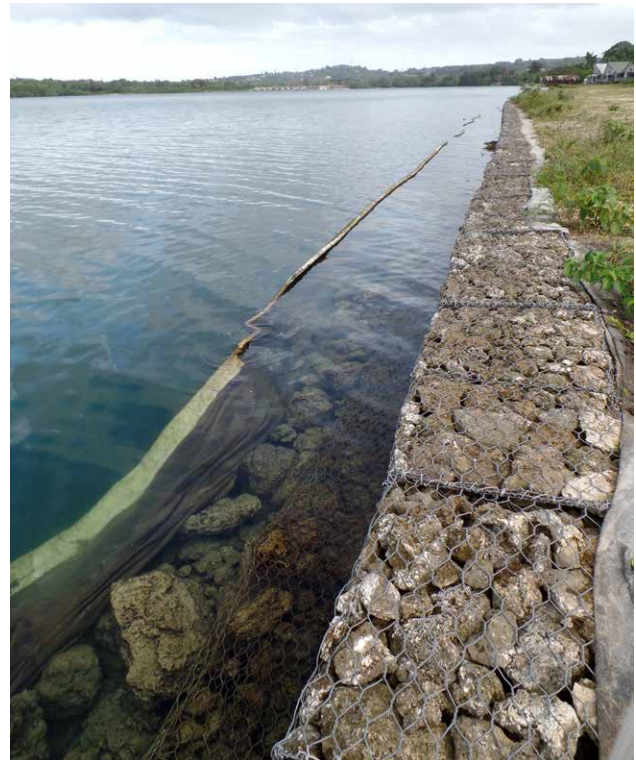
Coastal protection measures (e.g. seawalls) need to be carefully planned and assessed prior to implementation, to ensure they will effectively protect community assets and not cause unintended impacts along neighbouring areas of coastline. Photo: Melanie Bradley
