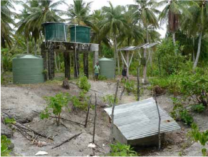
Plate33. Solar pump and water storage - from main well water supply for Vaitupu
