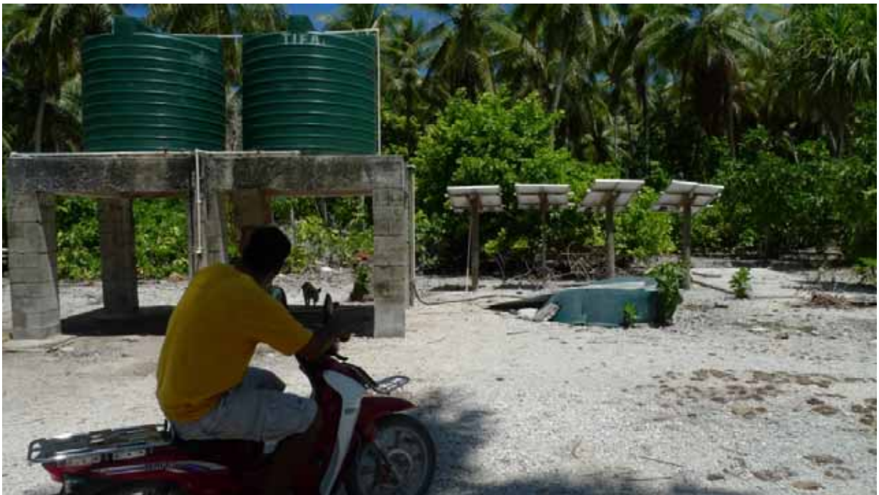
Plate 34.2 Communal Well - Nanumea with floating solar pump, not operating at time of survey. Salinity mS/cm approximately 1.5 km from village centre
