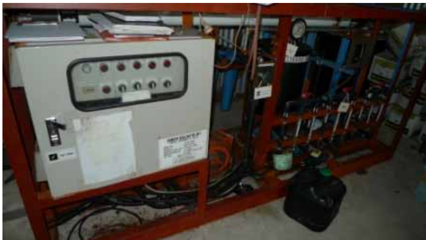
Plate 12 Desalination plant in Nanumanga- requiring refurbishment
