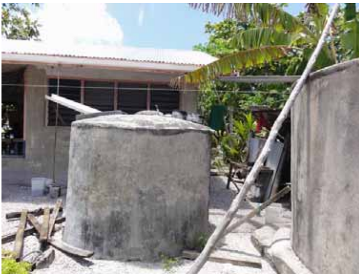
Plate 40. Rainwater harvesting - Niutao. Note the two concrete tanks, unconnected. When one tank is full the guttering is manually shifted to fill the other tank.
