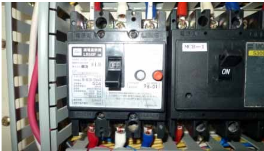
Plate 16 Main switch in control box
