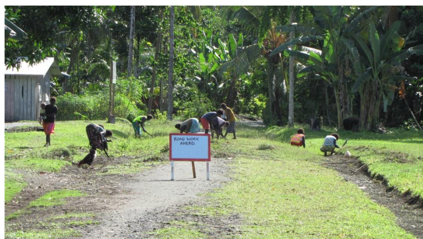
Women in the Solomon Islands (Choiseul Province) maintaining a road and verges for the SIRIP Project (ADB, 2010)
