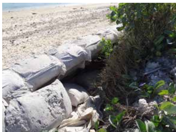
Photo 16: Overtopping (Credit: Shand)
