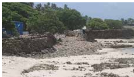
Photo 4: Stacked coral block wall in Kiribati collapses forming a 'dynamically stable revetment' (Credit: Shand)
