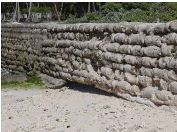
Photo 17: Undermining (Credit: Shand)
