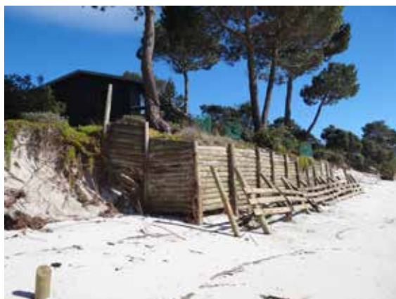
Timber pile retaining wall in New Zealand being undermined and outflanked (source: Shand, 2014)
