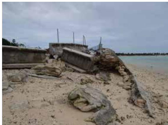
Photo 18: Structural failure (Credit: Shand)
