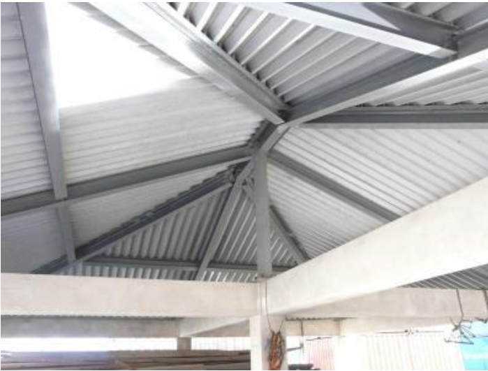
Photo: Roof space at container port building where myna have built a nest in the past
