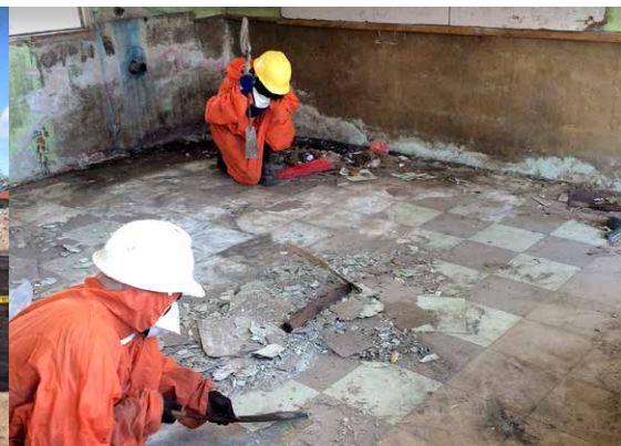
Asbestos removal works in progress at the site of the old Gizo Hospital. Photos: Brad Wallace and Don Hemmer.
