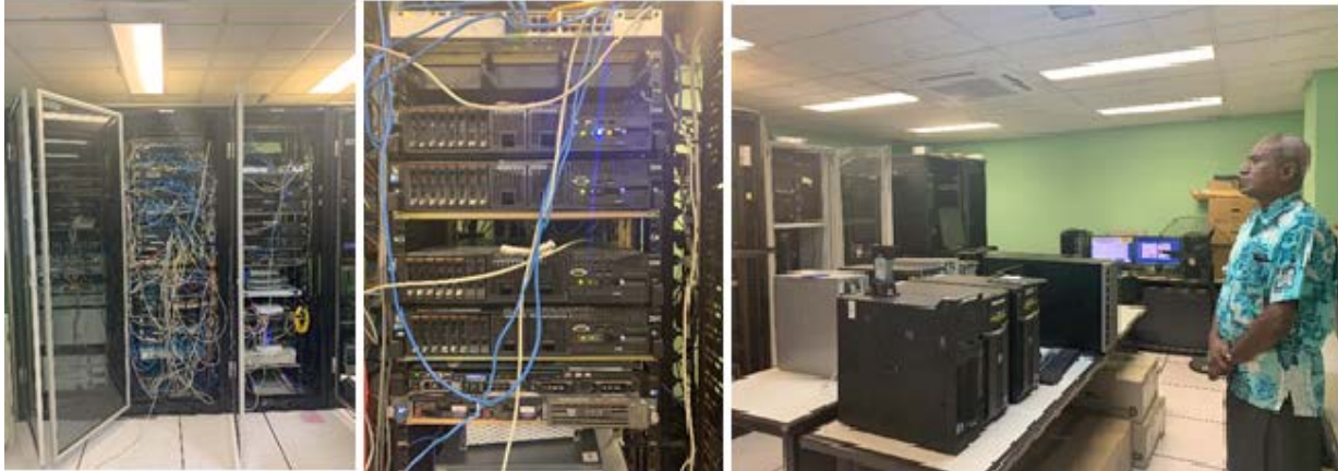
Figure 22. FMS's server room.
