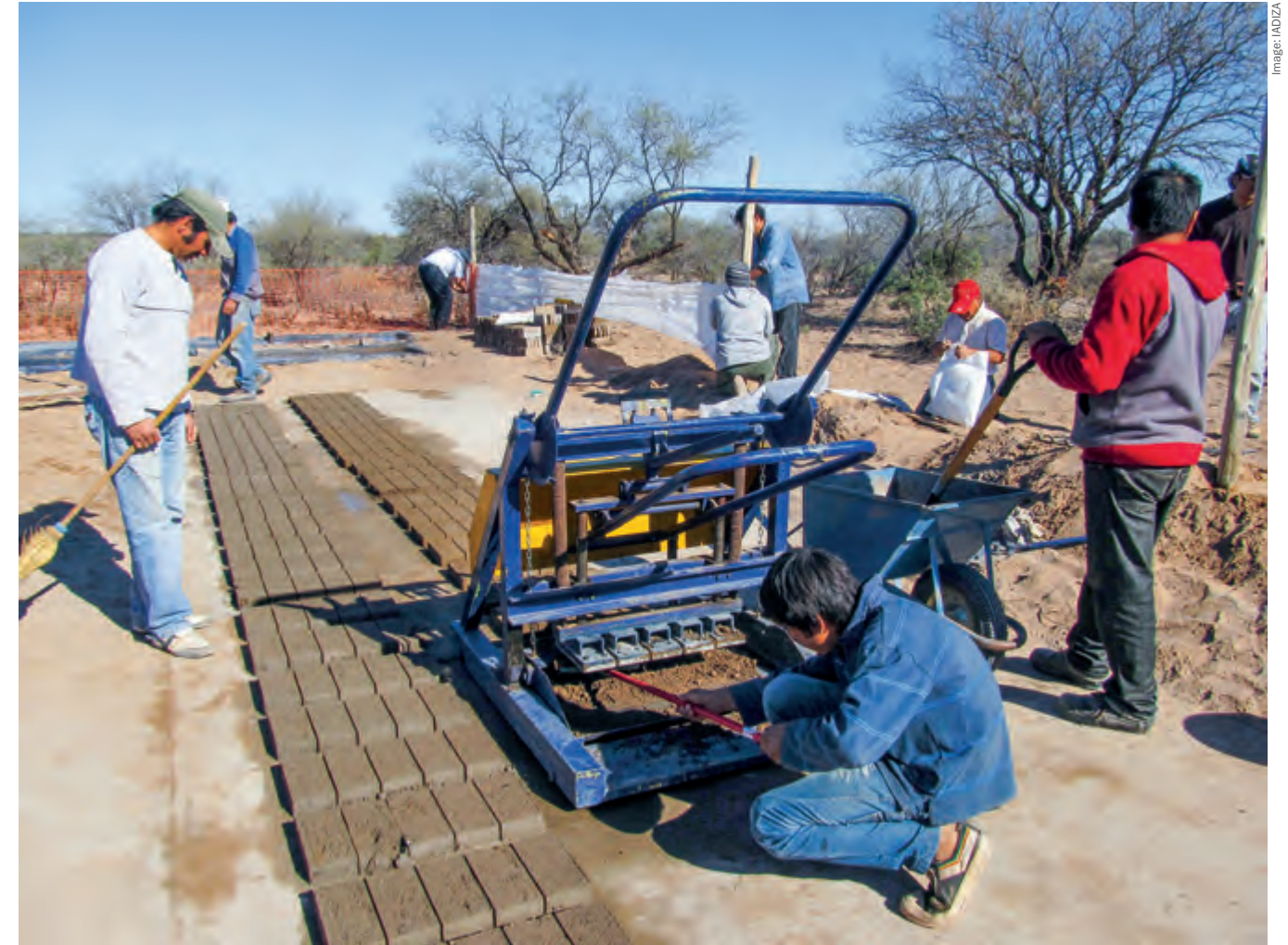
The community manufactures 'green' (unfired) bricks with local materials for the construction of the DPU
