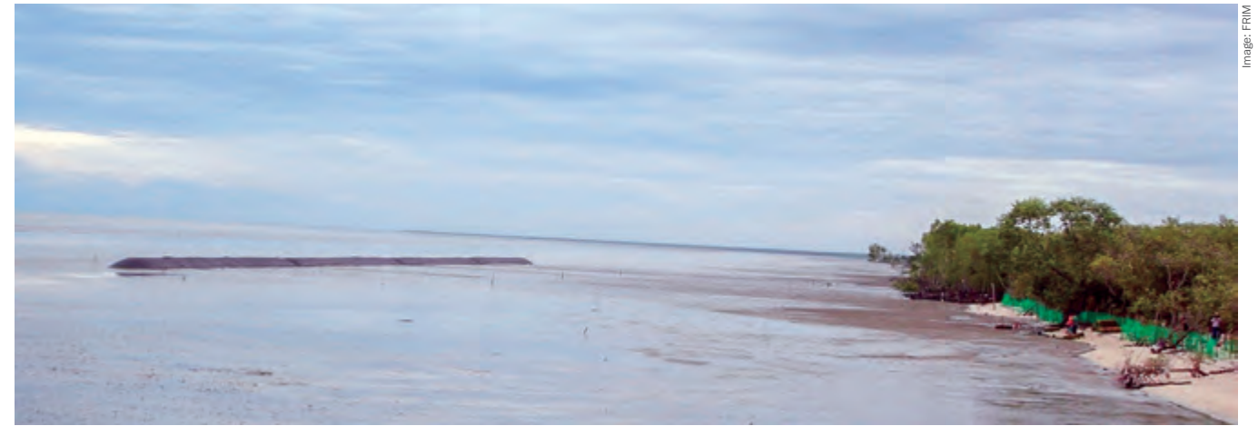
The geotube breakwaters constructed at the beach of D' Muara Marine Park Resort (before planting)
