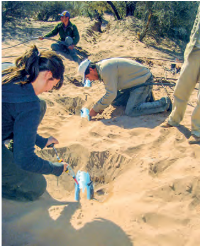
Construction of the water supply system for the DPU in the desert of Lavalle, Mendoza
