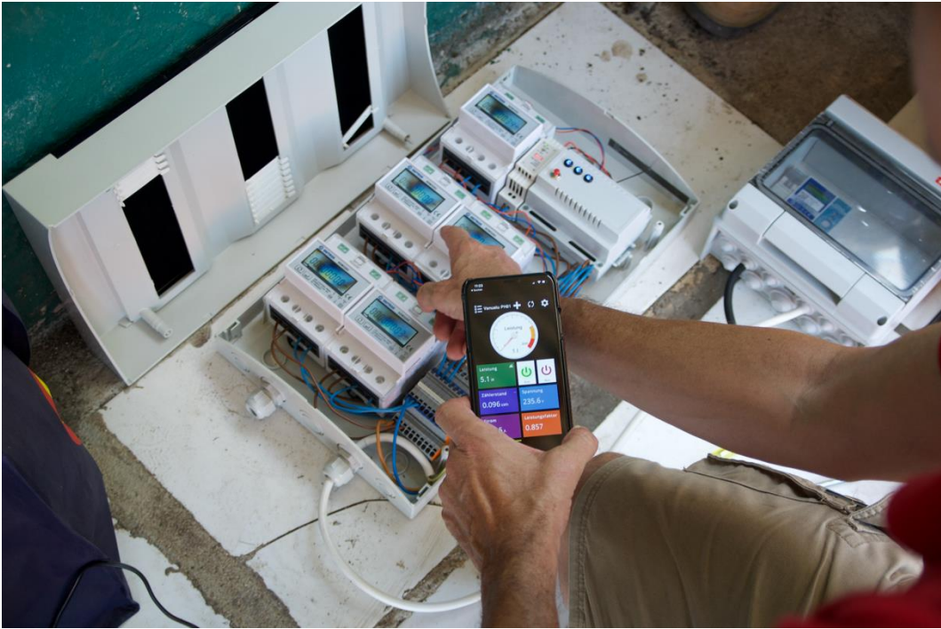
At the same time the Power-Blox were installed. This installation work consisted essentially of interconnecting the Power-Blox, connecting them to the central distribution switchboard and plugging in the solar modules.
