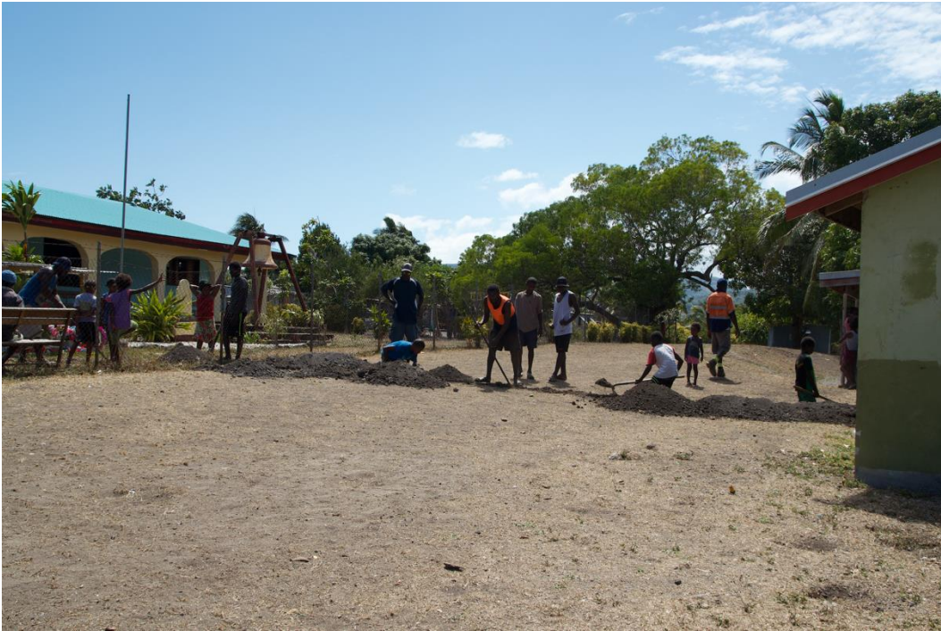
At the same time, the PCS team installed the solar modules and took care of the electrical interior installations of the first buildings.
