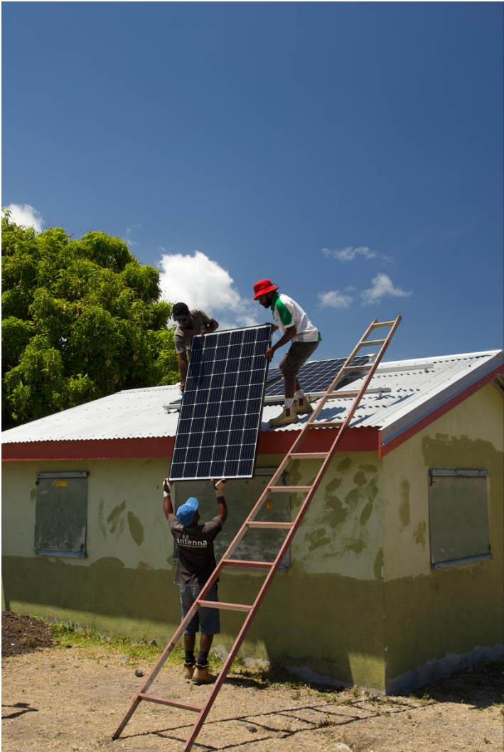
The buildings were equipped with basic infrastructure such as lighting, sockets and switches. Care was taken to install as much local material as possible, but at a good quality level. This with the background that the
