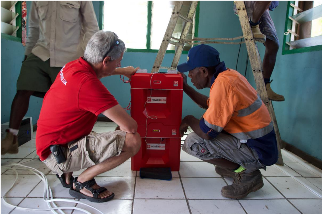
After the cabling work for the first two buildings was finished, these lines were already powered and tested.
