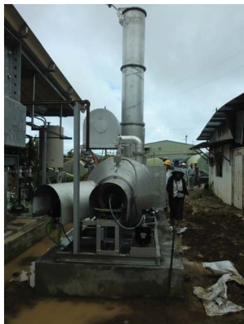
Figure 4-3 Waste oil treatment facility
