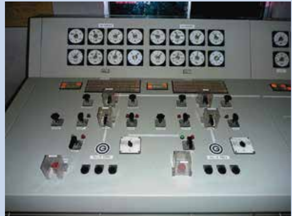
Figure 13: South Tarawa Bikenibeu power station control panel
