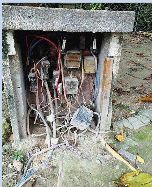
Figure 39: Pillar boxes and exposed cable terminations
