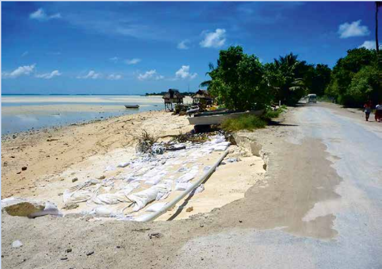
Figure 2: Damage to key infrastructure resulting from rising sea levels
