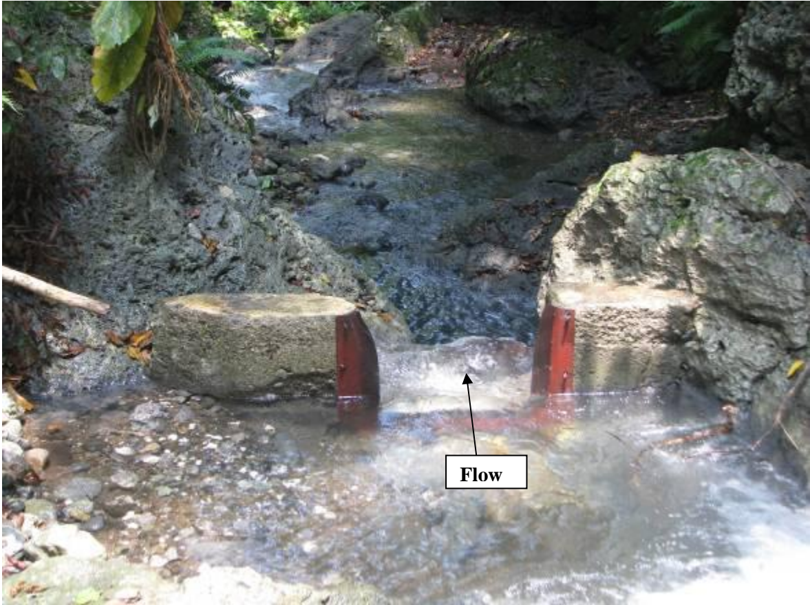
Figure 4-4 Huro Weir/Intake site
