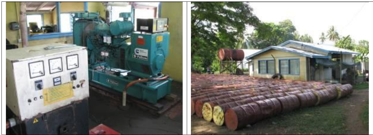
Figure 4-1 Kirakira Diesel Power Station
