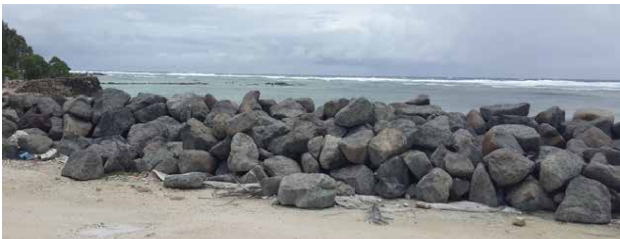
A sea wall recently reconstructed to protect a main road in Kiribati with Australian aid funding.
