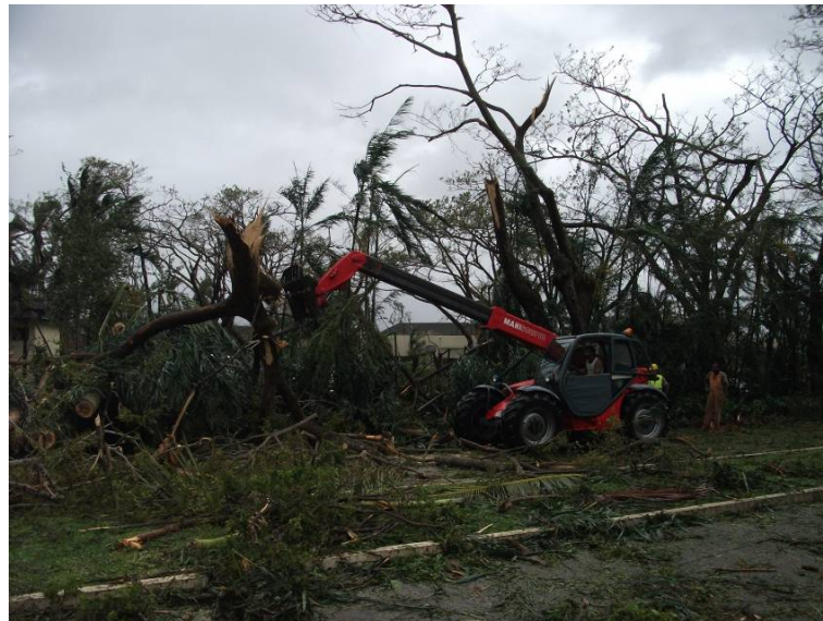
Figure 12. Clearing damage to vegetation in Fiji after cyclone Evan .
