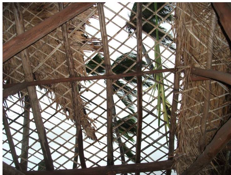
Figure 13. Damage to a roof of a traditional house in Nadi, Fiji Nadi, caused by cyclone Evan .
