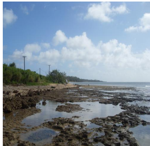
Coastal erosion west coast Foa Island, near the causeway.
