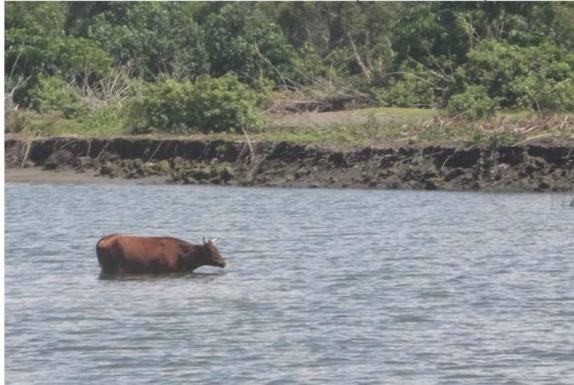
Bank erosion, Jordan River (Photo: L. Fatdal)
