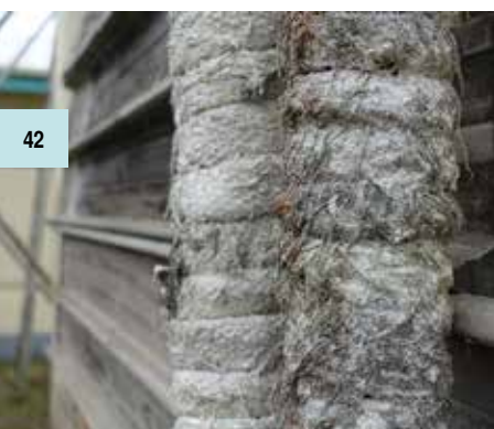
Asbestos rope lagging found during the PacWaste asbestos survey. Photo SPREP/E. Vanderburg
