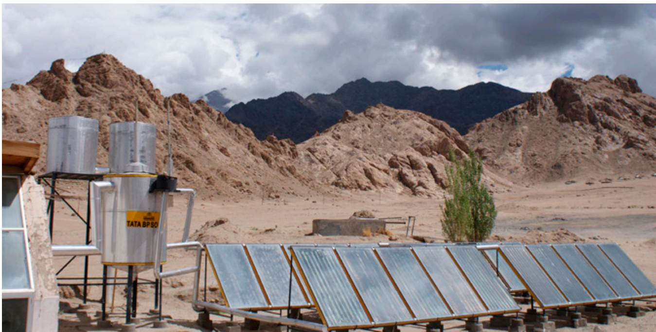
Water heating system installed in an area now recognised for its vast renewable energy resources. The use of these technologies ensures sustainability while reducing the long-term impact of developmental activities on the environment
