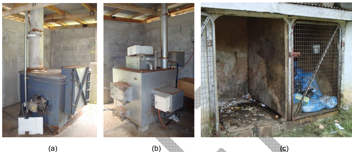
Figure 3: (a), (b) Incinerators located at the Port Vila Central Hospital; (c) medical waste storage area
