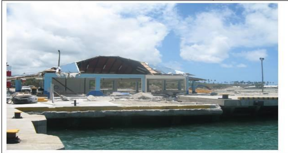
Figure Four-E: Aleipata Slipway and Wharf effect of Tsunami.
