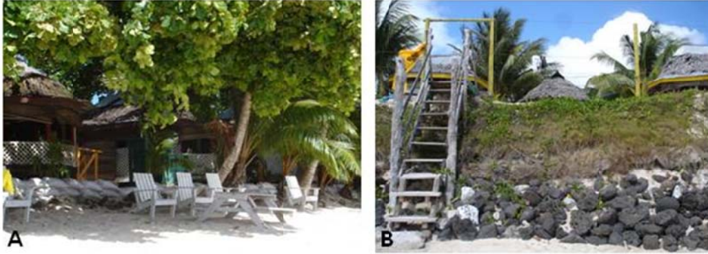
Figure 6. The Manase beach is impacted by hard-stabilization structures built to protect specific properties, including A) sandbags at Vacations Resort, towards the eastern end of Manase beach, and B) rock revetment at Tanu Fales, adjacent to the eastern edge of Stevensons Resort.
