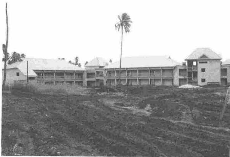
PLATE 2: Tourism development brings welcome economic benefits, but can have unwanted effects. Run off from construction sites, for instance, can lead to silt build up in local rivers or lagoons, damaging fishing sites, coral and other valued features of the local environment. These effects have to be anticipated and managed properly.
