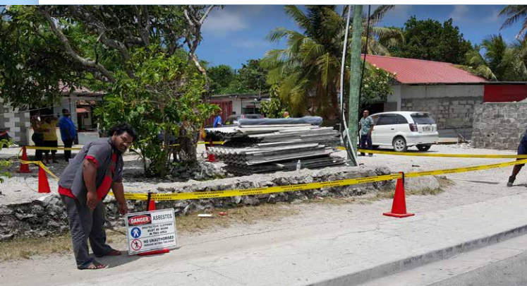
Participants practice setting up a safety cordon and signage in preparation for a practice asbestos removal activity. Photo: F.Griffin/SPREP
