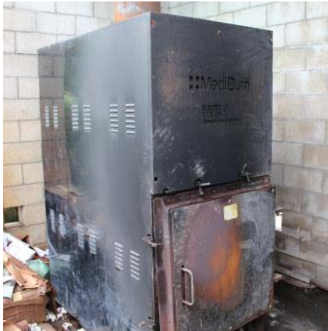
Photo 5: Figure 5: This is the operational incinerator at Tungaru Hospital. Photo taken on the 17/04/2014 by Trevor Thornton
