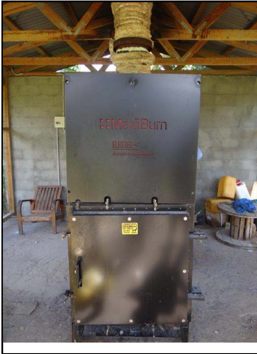
Photo 10: Second incinerator (MediBurn 20), Lautoka Hospital, Fiji (taken 24/3/2014 by Geoff Latimer ref:DSC03594)
