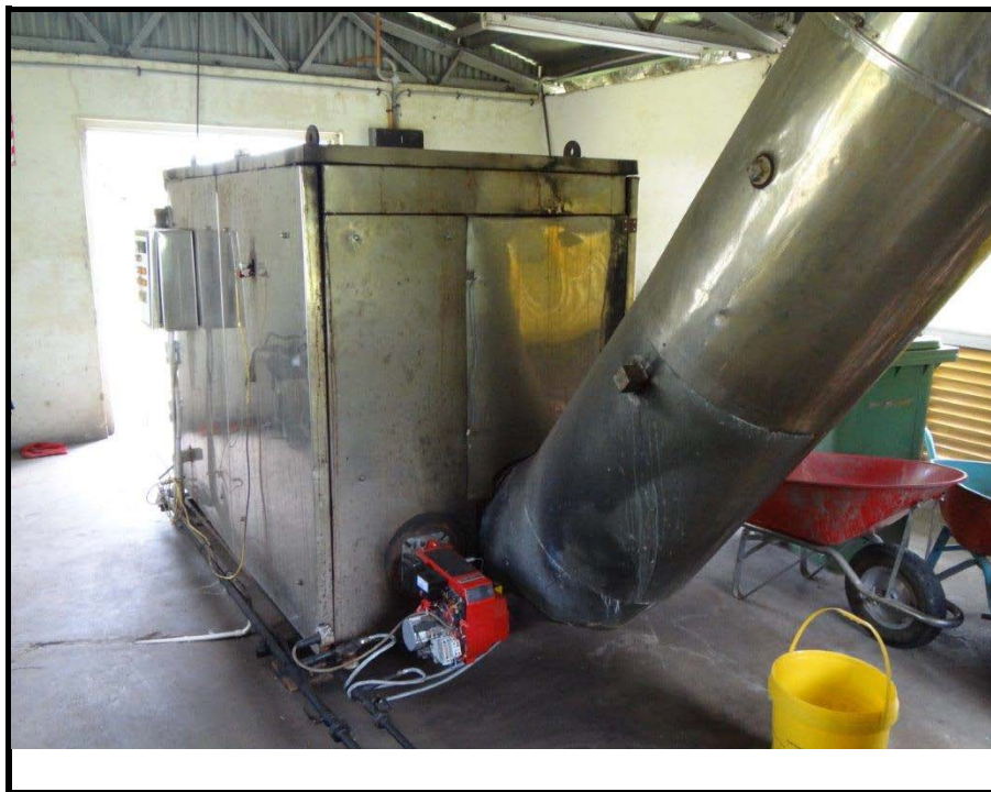
Photo 14: Main incinerator at Labasa Hospital, Fiji (taken 27/3/2014 by Geoff Latimer ref:DSC03758)
