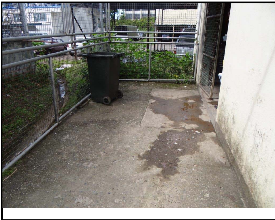
Photo 8: Pre-treatment storage area at incinerator building entrance, with open drain (left), CWMH Suva, Fiji (taken 26/3/2014 by Geoff Latimer ref:DSC03702)
