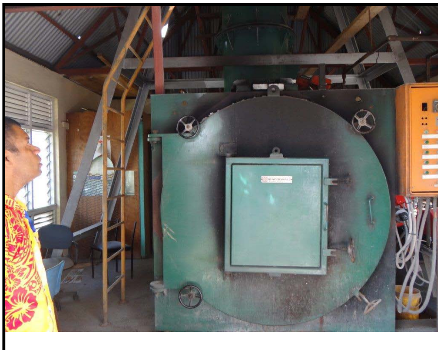
Photo 4: Incinerator, CWMH Suva, Fiji (taken 26/3/2014 by Geoff Latimer ref:DSC03696)
