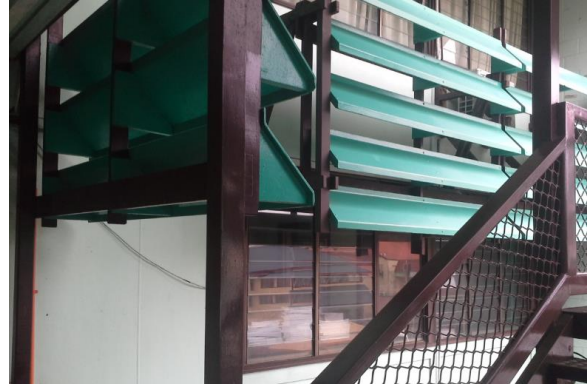
Photo 10 – WSLAC House Sunshades
