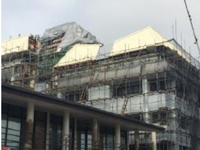
Photograph 7; View south west towards John Williams. Former roof (in green) being removed.
