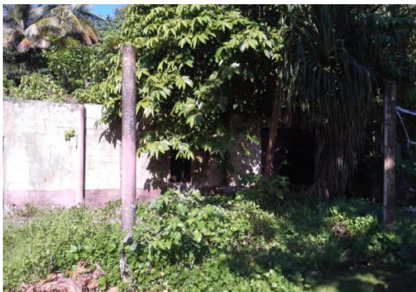
Photo 19 – Hospital – Old AC Columns
