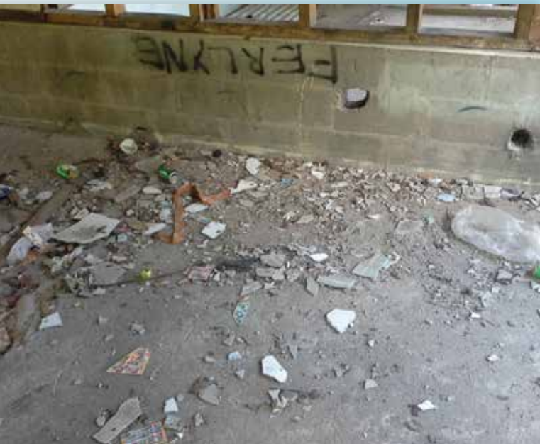
This vacant building in Nauru, littered with asbestos debris, appears to be frequented by young adults from the local community. Photo: PacWaste
