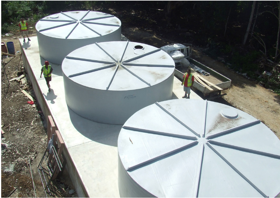
Figure 6. The ground level water tanks each with capacity of 45,000 litres.
