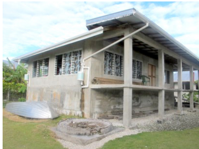
Figure 11. House with new guttering and two FFDs connected to under-house concrete tank. (Photo: PACC+ project.)
