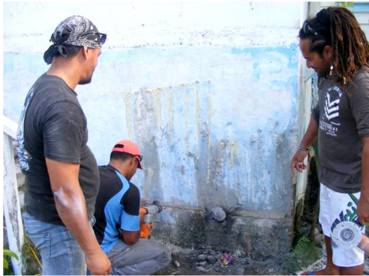
Figure 10. Kiara plumbers with the Nukunonu PACC+ focal point Mr Mikaele Maiava supervising the tank repair activity. (Photo: PACC+ project.)
