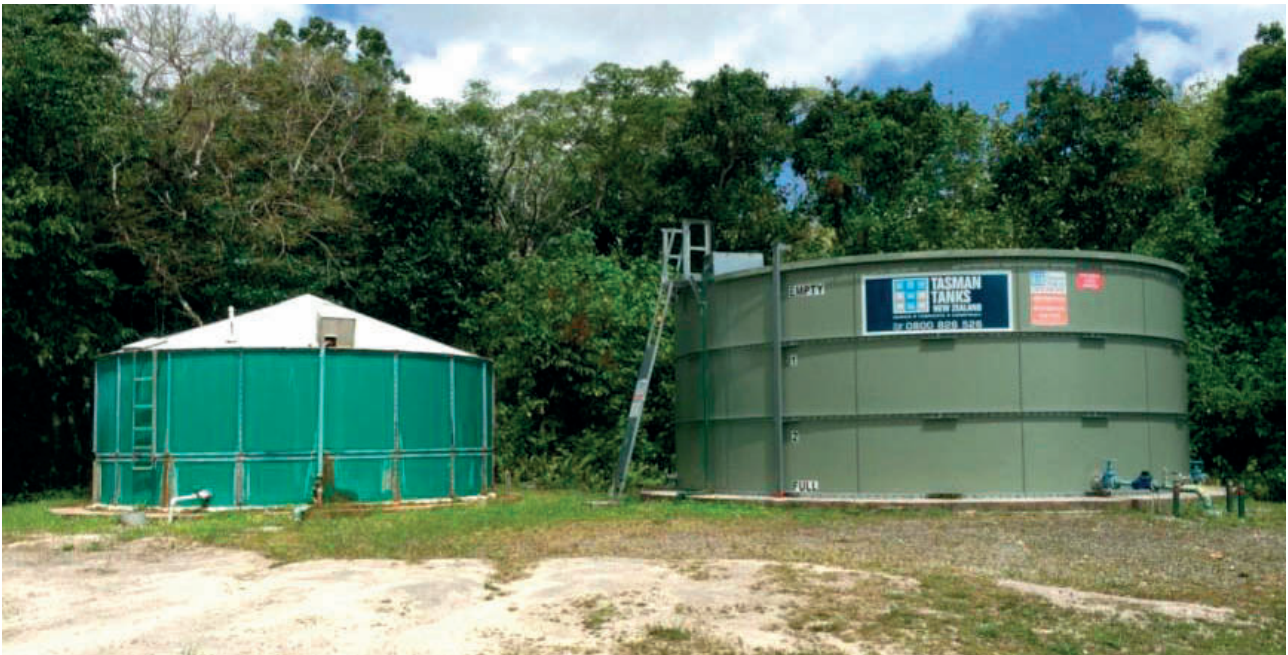
Figure 5. Storage tanks (old on the left and new on the right) in Tamakotoga. (Photo: Niue PACC Project.)
