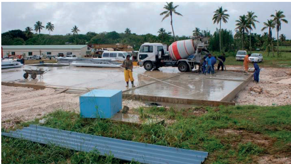
Figure 13. Building the foundations for the tank moulding factory. (Photo: Niue PACC Project.)
