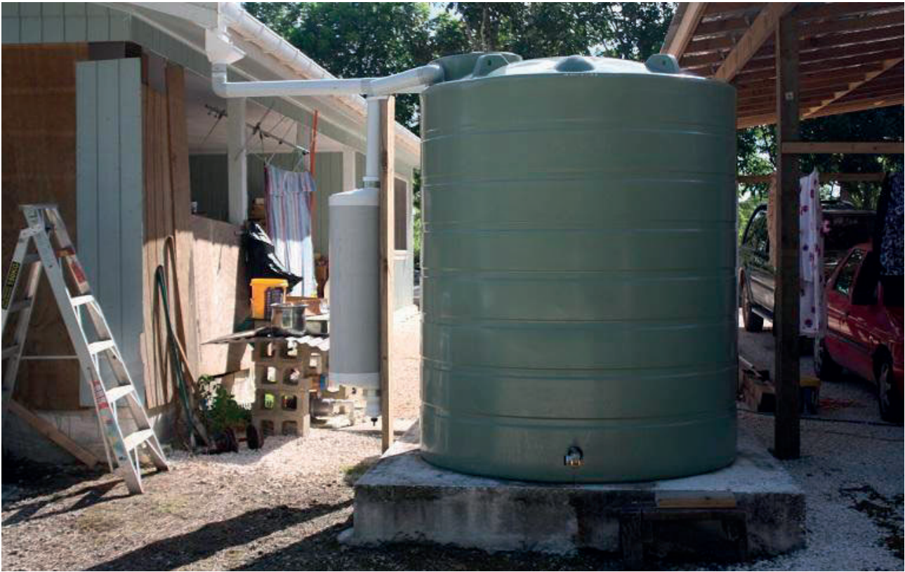
Figure 18. Installed rainwater harvesting system.
