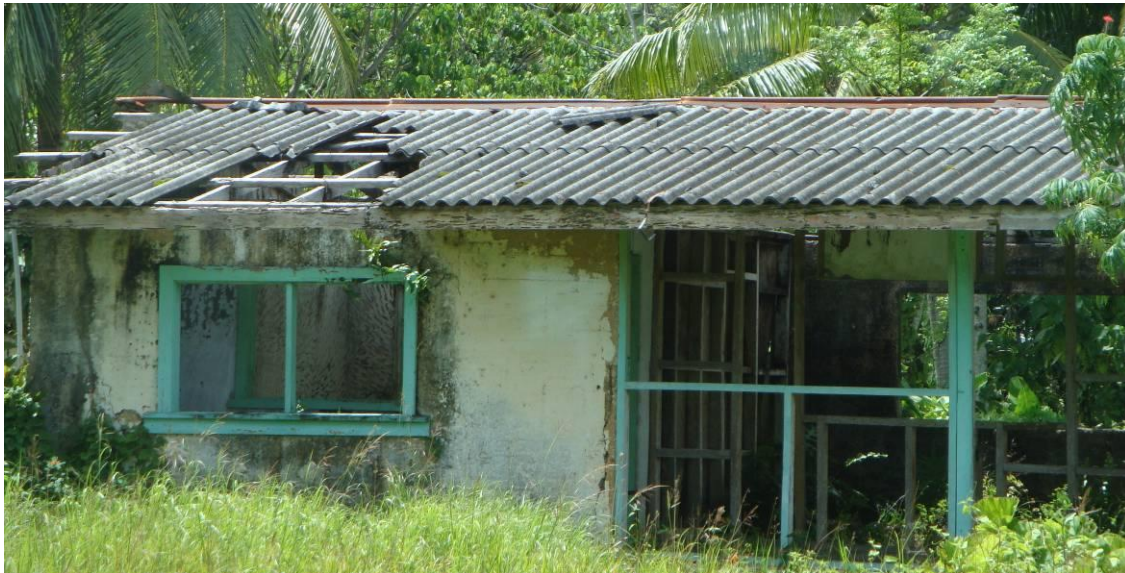
Picture 5: Typical abandoned house with asbestos roof sheets
