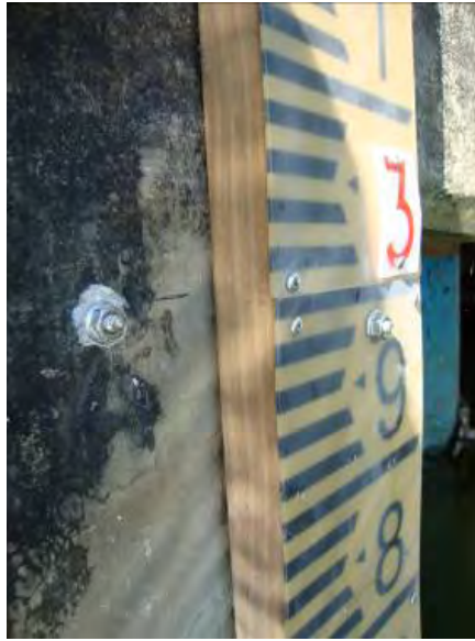
Figure 2-5: Backup external reference point is the top of the threaded inner shank of the dynabolt. This has a recorder level of 3.0 m. A tape measure can be used to measure water level from this point if the staff gauge plates are lost.
