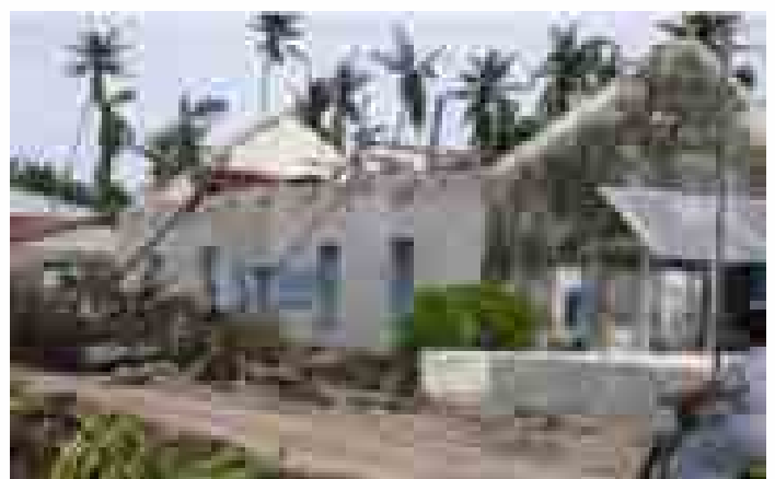
Damaged building in Pukapuka after TC Sally 2005
