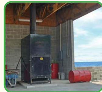
Regular maintenance of equipment is critical to sustainable healthcare waste management.
