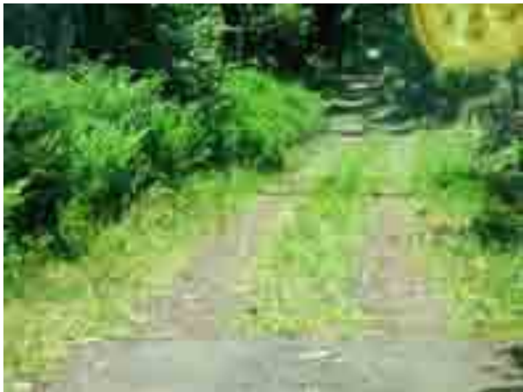
Unsealed access road with poor drainage
