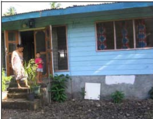
A raised threshold prevents damage from minor flooding.
