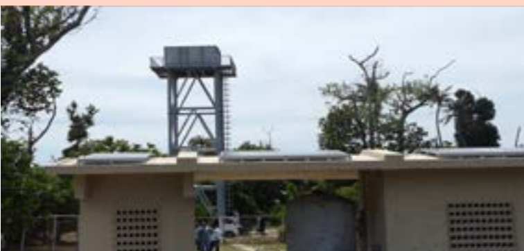
The new Kayangel Island Solar_PV water pumping and supply system, has replaced the electric motor driven pumps of the Kayangel well water systems. Photo A. Abraham.
