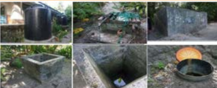
Existing water tanks and wells from outer islands like those pictured from Eauripik, Woleai atoll, Ifalik, and Feraulap atolls are often in poor conditions.
